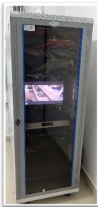
Sulthan Gold – CCTV and Networking
